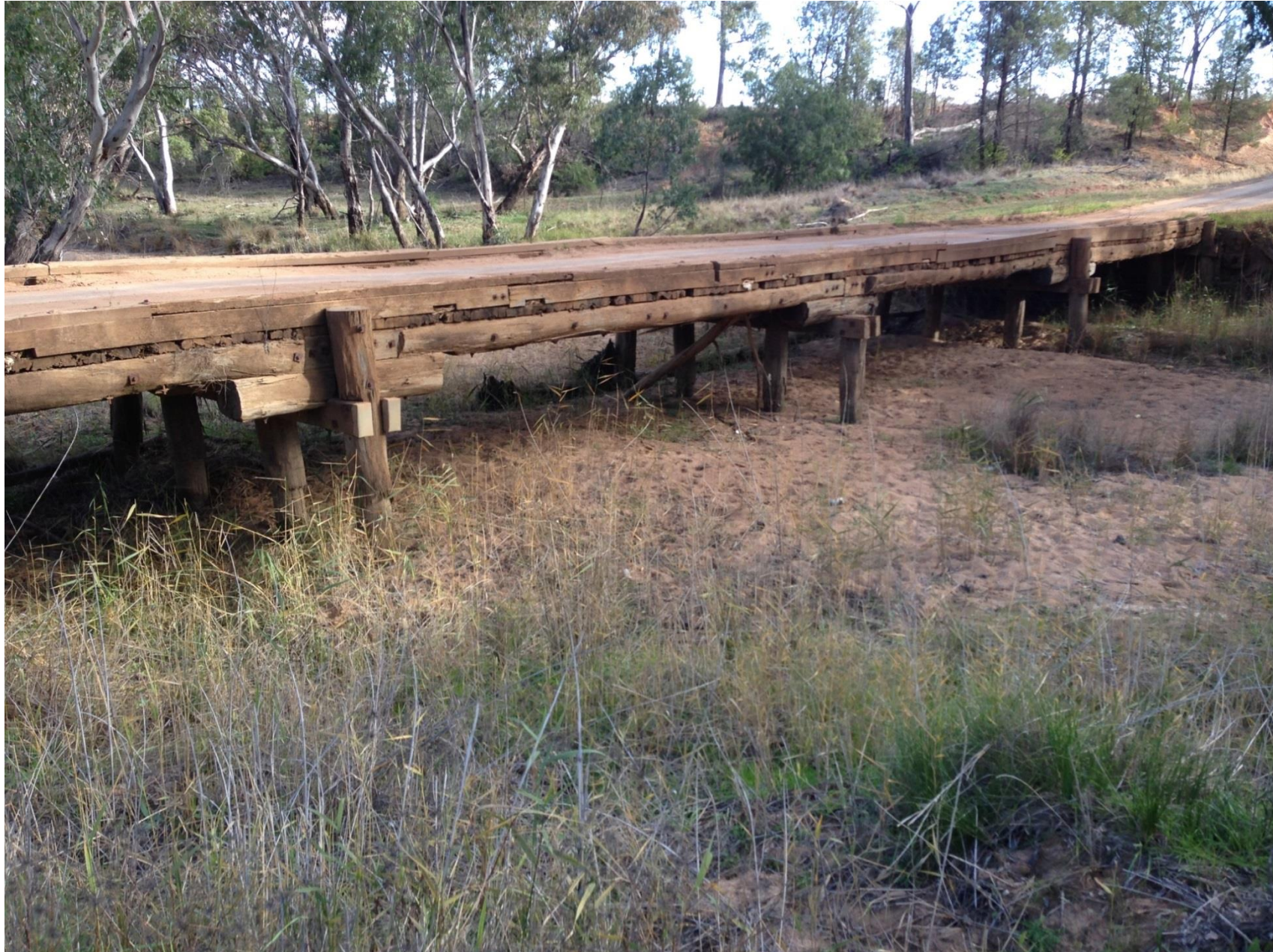
Side view photograph of bridge over Baradine Creek near the Village of Kenebri.
